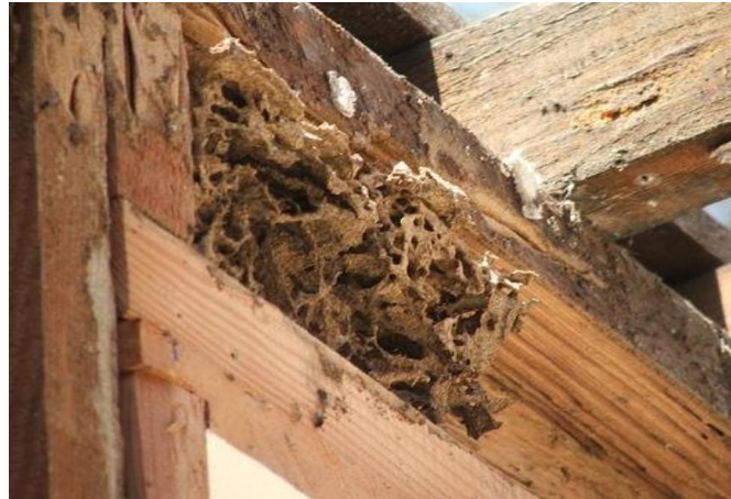
Figure 2: Termite Damage on Building Structure [5]
