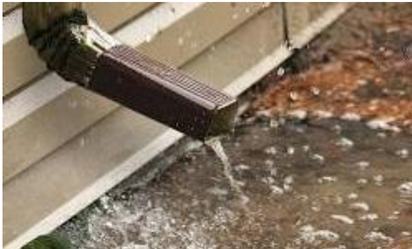
Figure 2: Unmaintained gutter overflowing water on house foundation [2]
