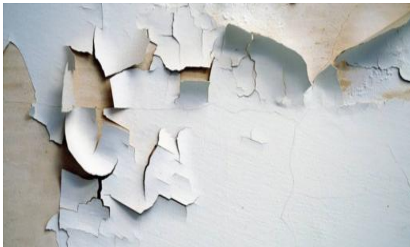
Figure 1: Peeling paints from the wall [1]
