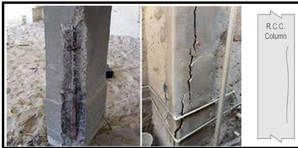
Figure 4: Corrosion Crack In The Concrete Column [3] [4]
