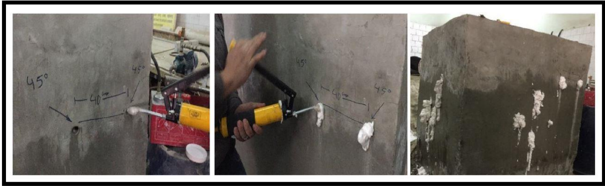
Figure 4: PU Injection To Repair Water Tank Crack [4]
